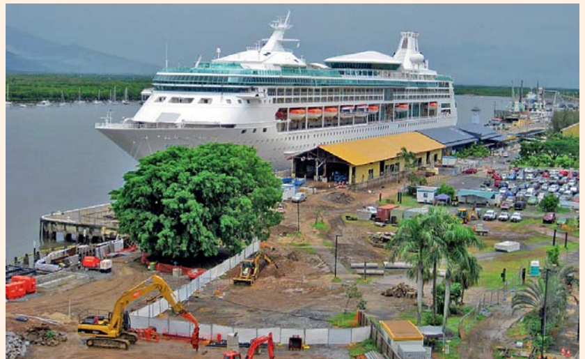
Hutchies has begun work on the $23 million works to complete the 1.6 kilometre public waterfront promenade linking the Esplanade through to the new Cairns Cruise Liner Terminal.
